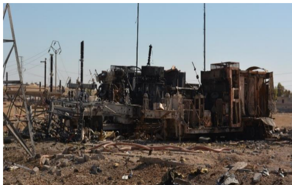
JCC Photo 7: Mobile generator burnt
